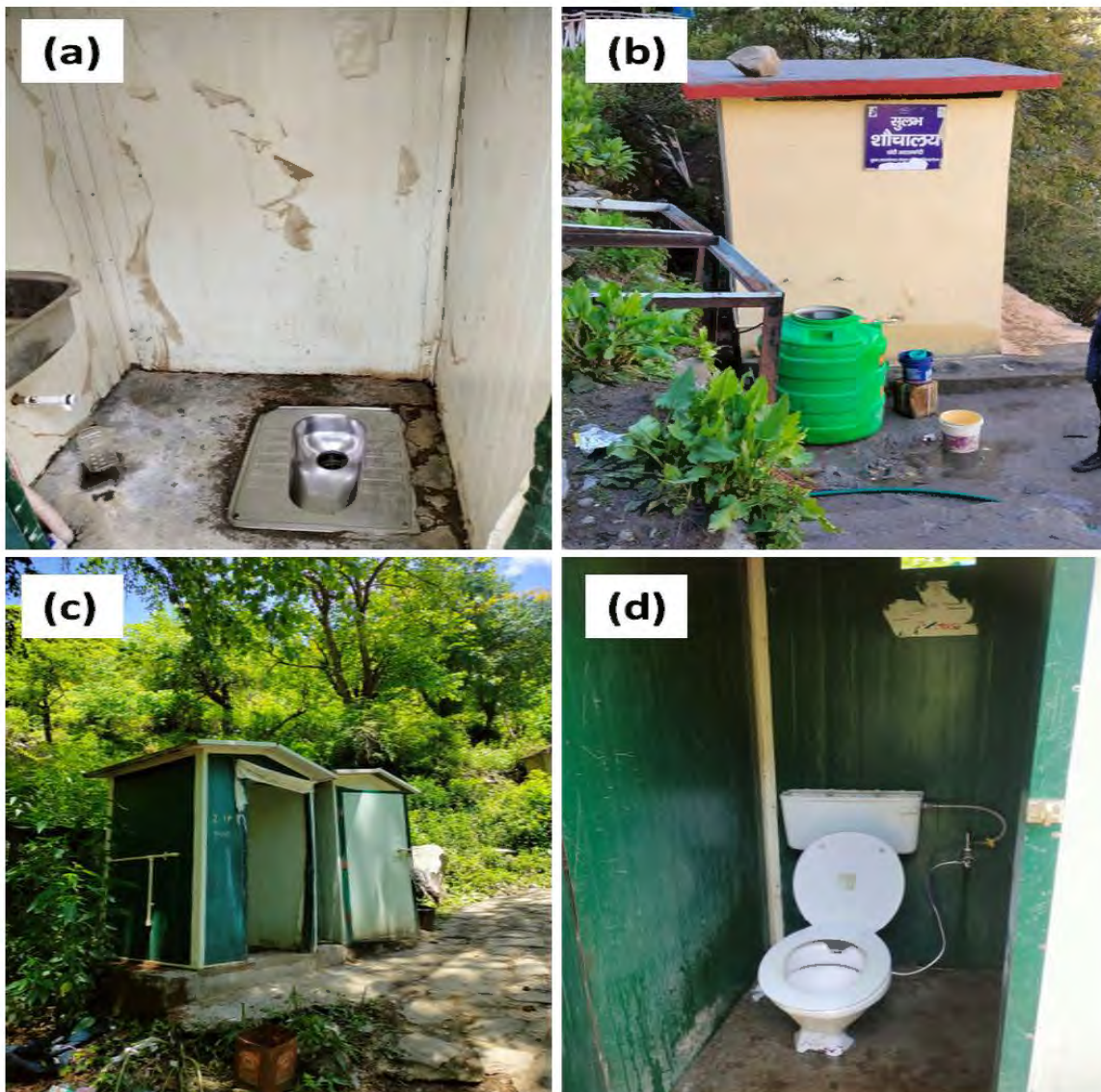
Plate 3.1.5: Sanitation condition (a) Poor hygiene, (b) Sulabh toilet, (c) No door structure, and (d) Poor maintenance
